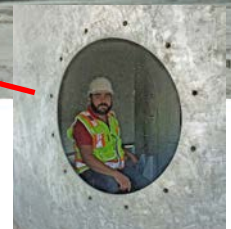
Inside the Suction Header
